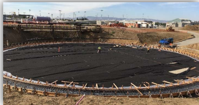
Non-Potable Storage Facility
