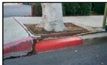
This sycamore tree has outgrown its planter and is damaging the sidewalk and curb.
