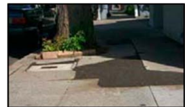
Severely damaged sidewalks such as this can be hazardous to pedestrians and costly to repair.
